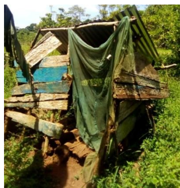
Figure 9: Example of household latrine that needed to be improved
